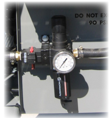
Figure 28: Air control system- trap and gauge
