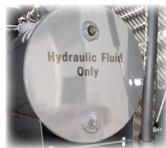
Figure 27: Hydraulic fluid reservoir
