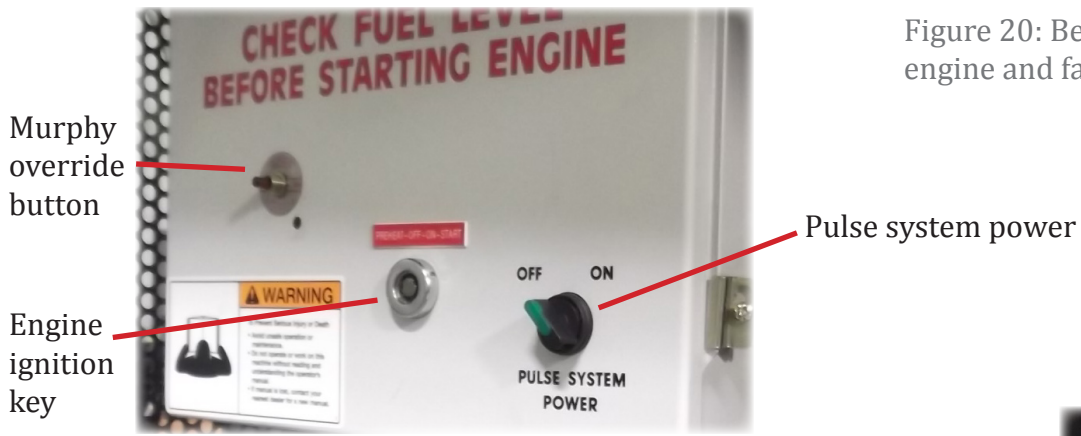
Figure 21: Main control panel
