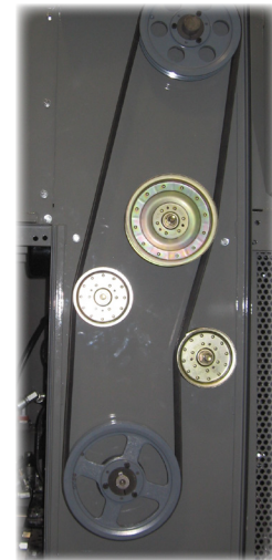
Figure 25: Fan drive belt on diesel engine
