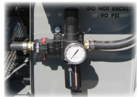
Figure 19: Shut off valve, regulator, and filter for pulse system
