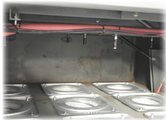
Figure 33: Pulse system inside filter bay.
