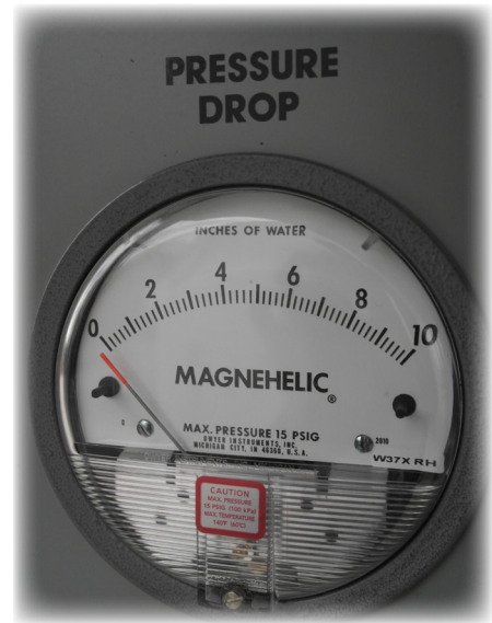
Figure 7: Magnehelic gauge displays restrictions in filters
